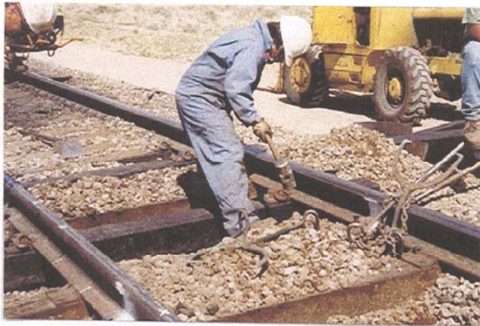
Figure 3- Recycled Plastic Composite Ties Being Installed at AAR's FAST Track in Pueblo, CO.
